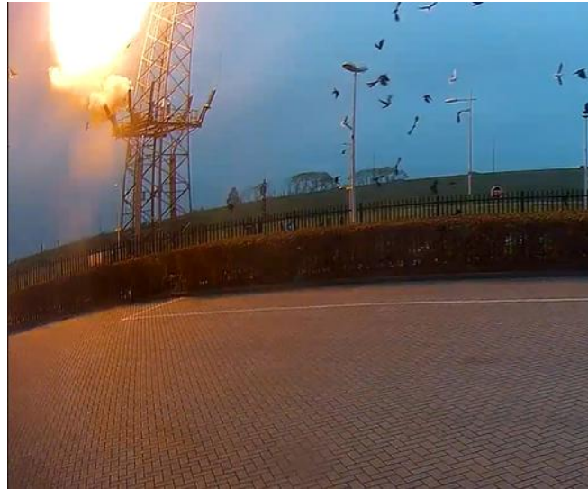
Figure 30. Fault in the cable section of the mixed circuit
