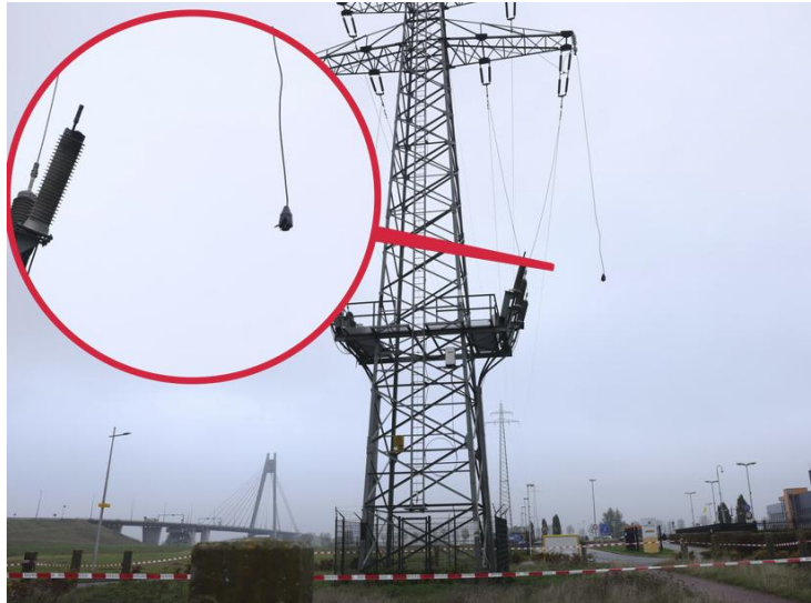
Figure 32. Destruction of the affected circuit equipment
