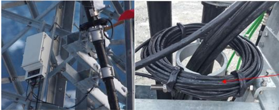
Figure 20. Low-power instrument transformer with dimensions 26.3 x 62.5 x 15.3 cm, weighing a total of 10 kg
