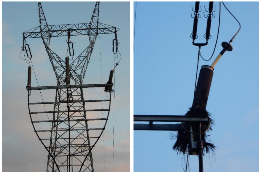
Figure 25. Pylon of a 220 kV mixed line with a damaged termination on the phase on the right side
