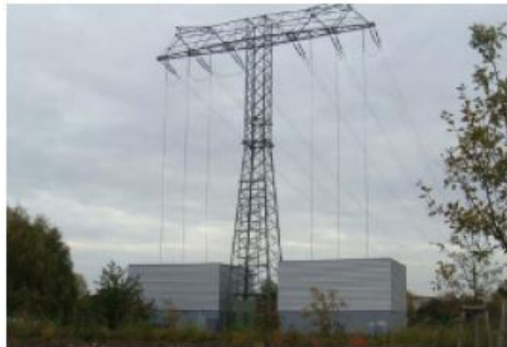
Figure 29. Implemented solution over the affected UGC–OHL crossing [14]
