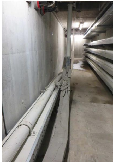
Figure 24. Destruction in the cable canal
