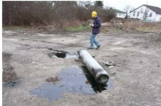
Figure 28. Pollution and damage to neighbouring properties caused by the explosive fault [14]
