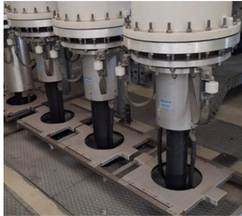
Figure 56. Example in the substation using a Rogowski coil
