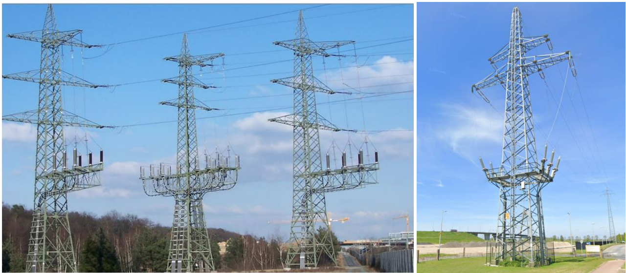
Figure 16. Different types of towers with a transitional point
