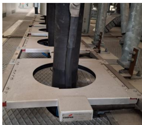
Figure 21. Rogowski coil application for measuring current on a cable section
