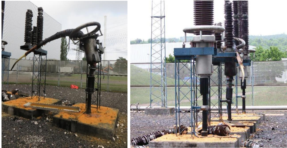
Figure 22. Destroyed cable after a fault in the termination
